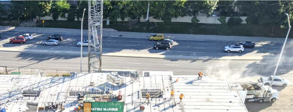
The Kay, a 128-unit development, is expected to be completed in early 2022.
